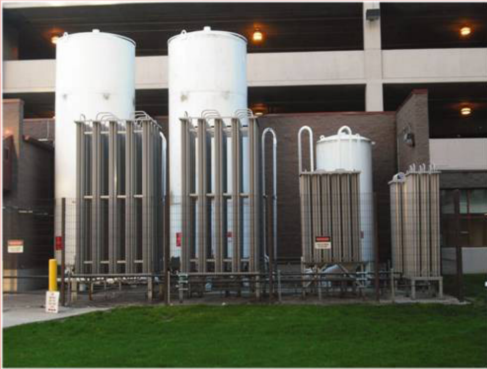
Liquid oxygen installation (Source: http://rc.rcjournal.com/content/58/1/173 )
